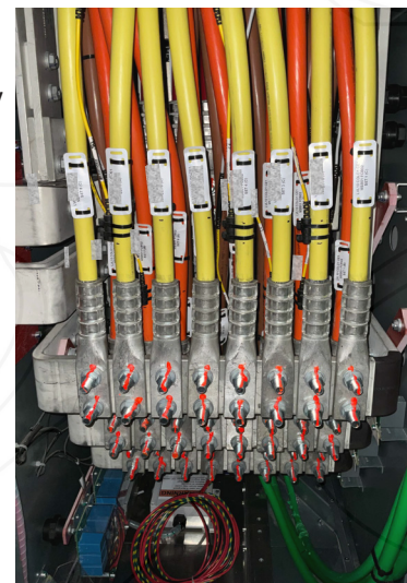
Bellevilles installed on bolted terminals
